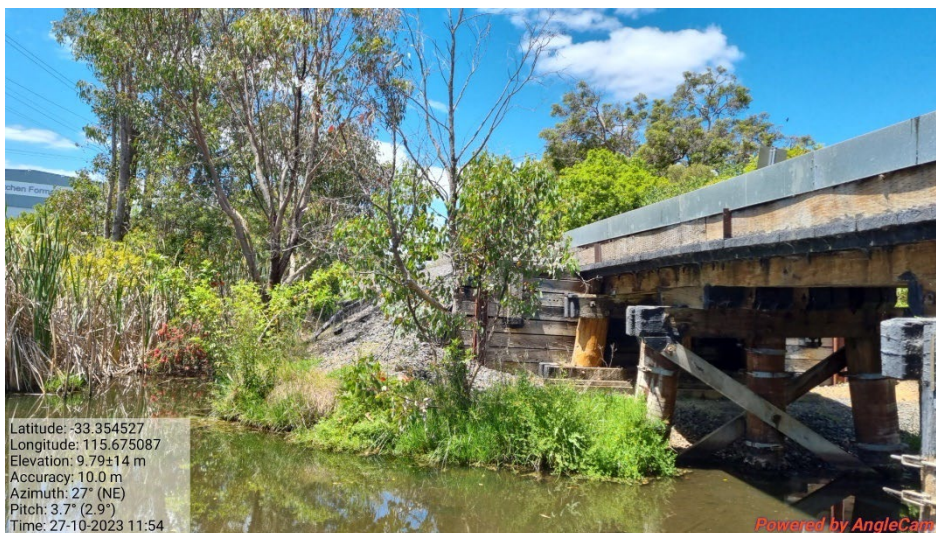
Plate 2: Vegetation within the Dodson Road Bridge Survey Area, Bunbury. Top: southwest bank. Centre: southeast bank. Bottom: northeast bank.
